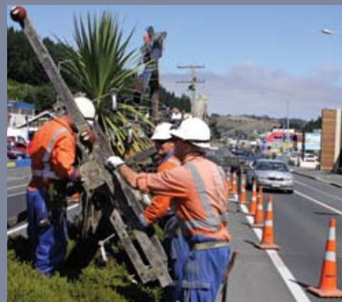
Overhead lines are removed from Dunedin's Kaikorai Valley Road, improving aesthetics and road safety.
