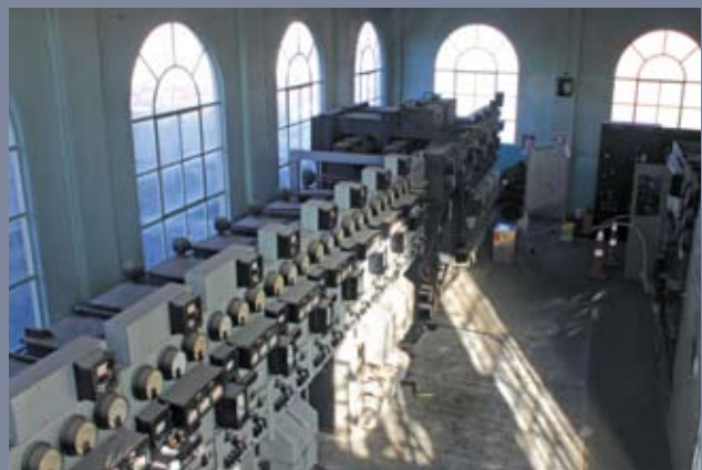
Built in 1938 in art deco style, the Ward Street substation was upgraded with heritage conservation a major objective of Aurora's asset management programme.
