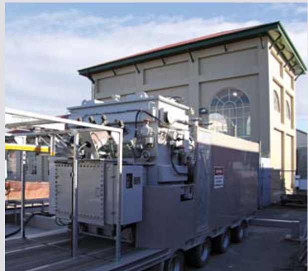
Aurora's mobile substation provided temporary service while the Ward Street substation was upgraded.
