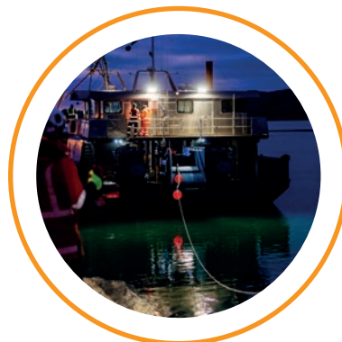
The Patiki Barge was custom fitted and transported from Picton especially for this project.
