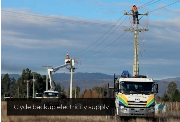
Outram zone substation upgrade
