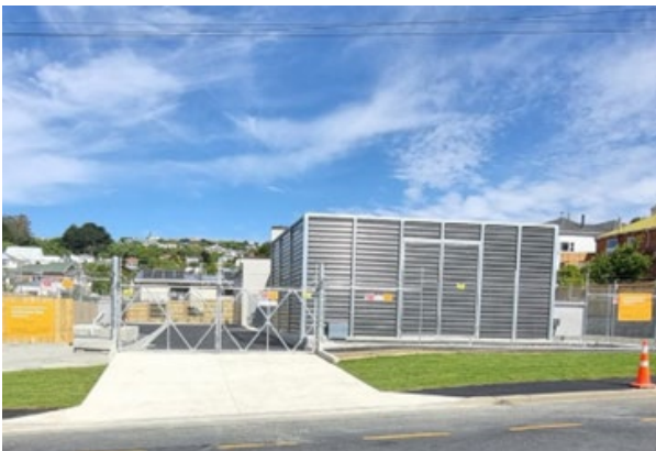
Figure 11-28: Andersons Bay zone substation
