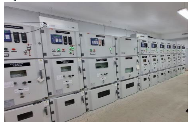
Figure 11-35: Indoor switchboard at Andersons Bay
